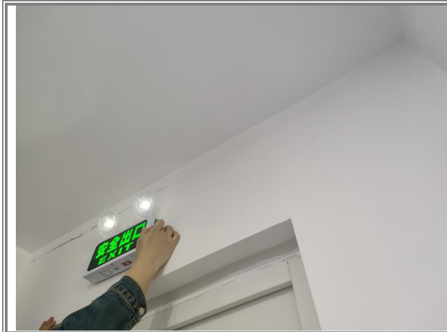
Emergency light test
