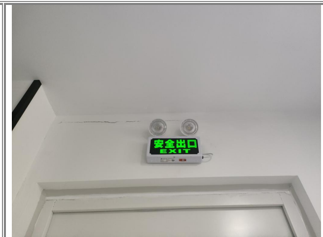
EXIT sign, Emergency light
