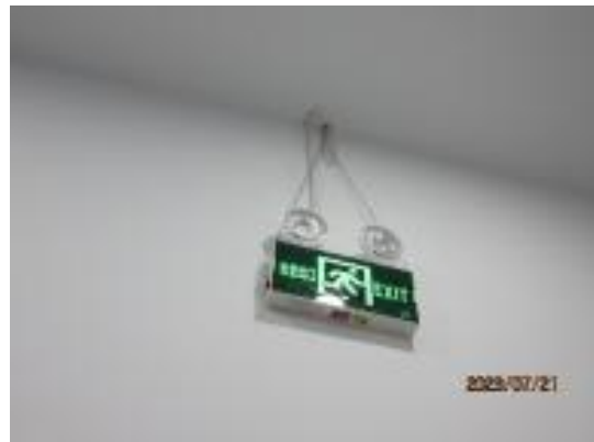
safety exit sign and emergency light.JPG
